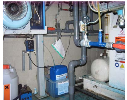
Before Installation: liquid chemical dosing point
