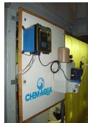
After installation: HandiChem System for cooling tower treatment
